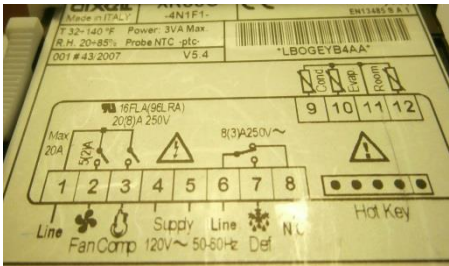
Freezer Controller Terminals
